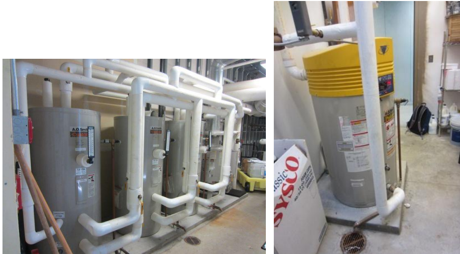
DHW storage tanks and heater
