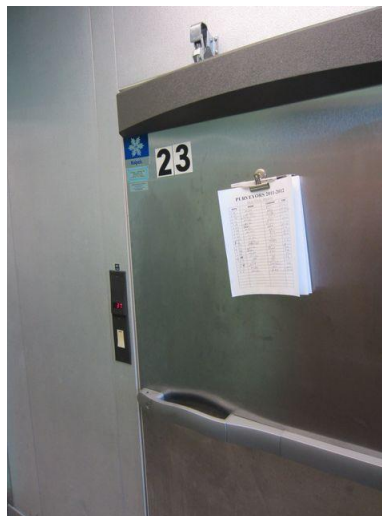
Walk-in refrigerator and freezer
