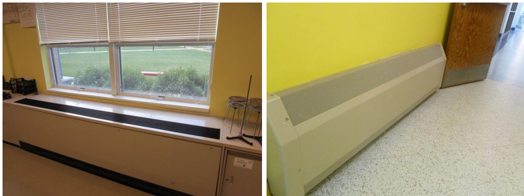
Typical classroom unit ventilator (L) and typical baseboard heater (R)
