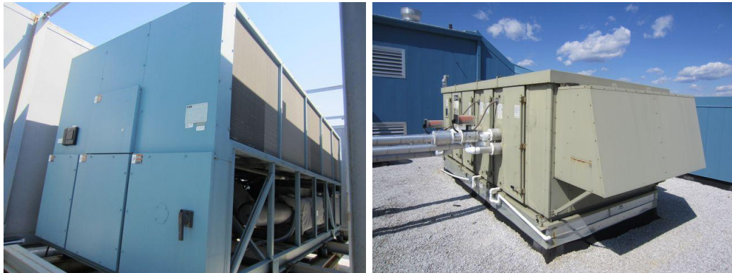
Trane air cooled chiller (L); typical rooftop (R)
