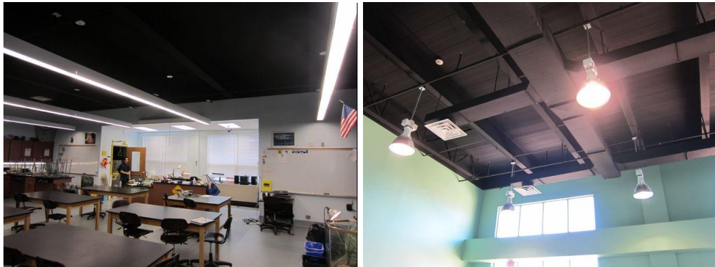
Typical interior classroom T8 lighting (L); and high bay metal halide lighting in the cafeteria (R)
