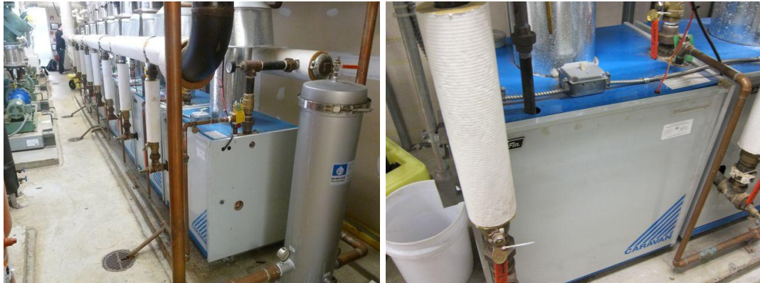
Slant/Fin Caravan Boilers
