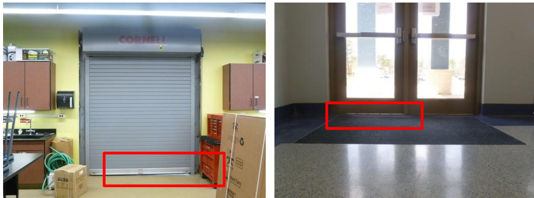
Deteriorating weather-stripping on Flex Lab roll-up door (L), and a main entrance door (R)
