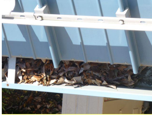
Foliage in gutters may lead to poor drainage
