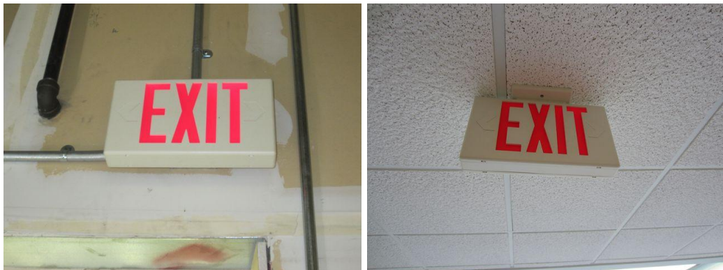
Typical old (L) LED exit signs
