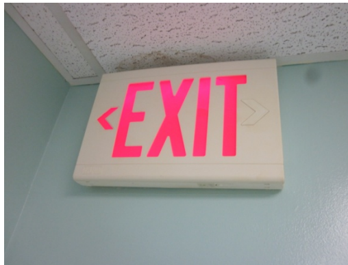
Typical LED exit sign
