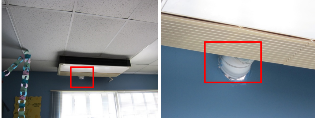
Poorly sealed wall penetration
