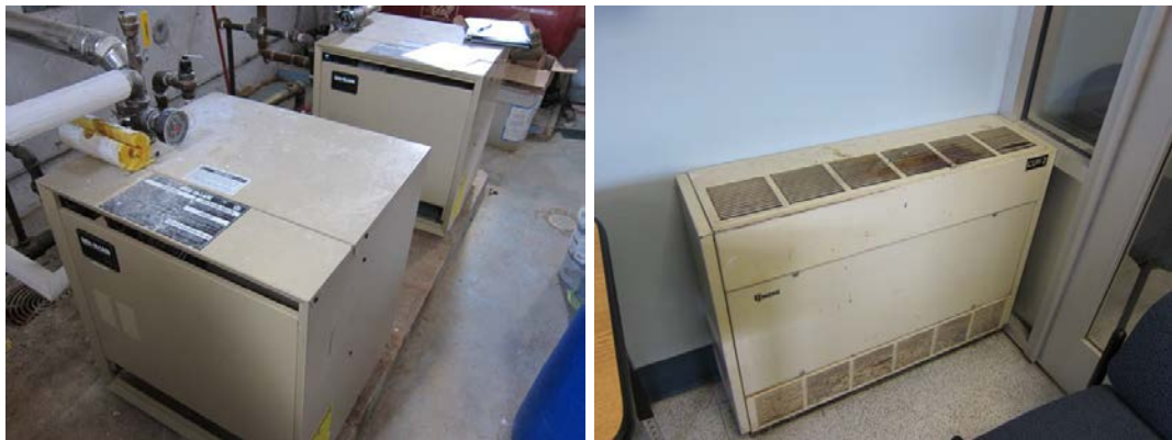
Two 233 MBH Weil-McLain Boilers (L), typical cabinet unit heater (R)
