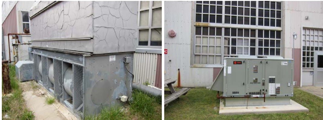
Evapco cooling tower (L); Trane outdoor packaged unit (R)
