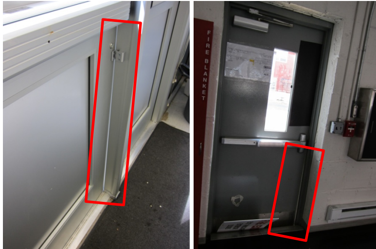
Metal doors have non-insulated door frames, and outside light shining through is a sign of no or deteriorating weather-stripping
