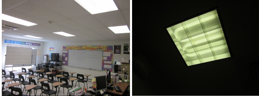
Typical interior T8 lighting (L); and typical T12 U-shaped lighting (R)
