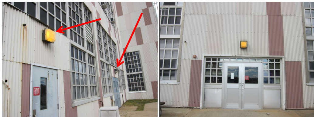
Typical high pressure sodium wall pack fixtures. Note: Some of the fixtures are operating during daytime hours
