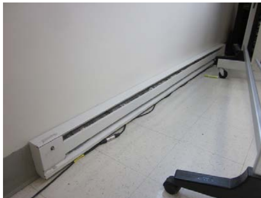
Typical electric baseboard heater
