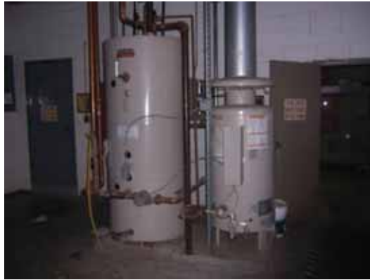
Domestic water heater and storage tank in original boiler room
