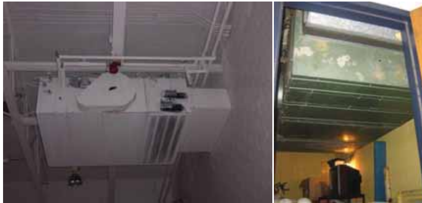
Typical H&V unit serving the main gym (Left) and AHU serving the associated locker rooms
