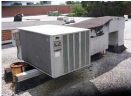
Trane RTU serving media center offices
