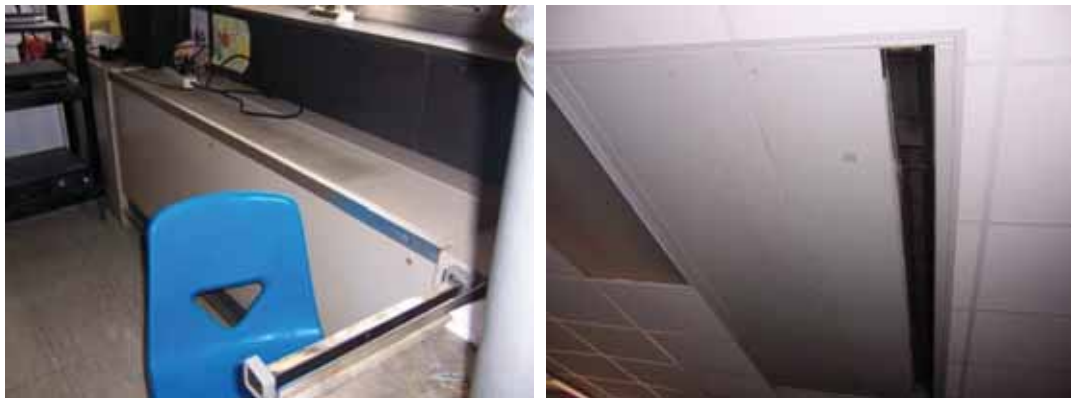
Examples of floor-mounted (Left) and ceiling-mounted hot water unit ventilators in the E-wing
