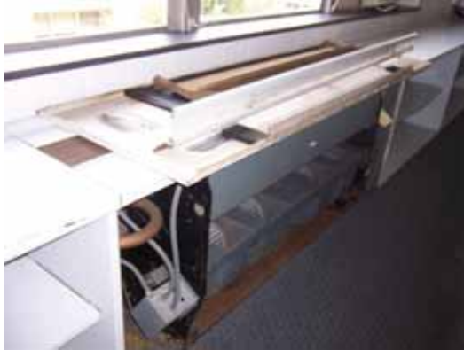
Example of the floor-mounted, hot water unit ventilators serving the A-wing classrooms
