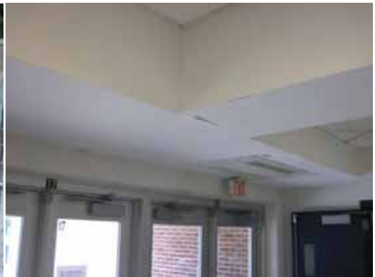
Water damaged gypsum wallboard visible in the interior
