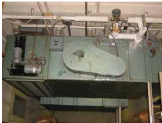
One of (2) AHUs located in the wood storage room serving classrooms B107 and B109
