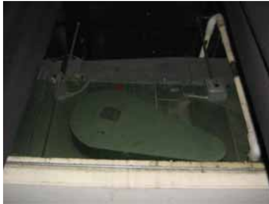
One of (2) H&V units serving the auditorium
