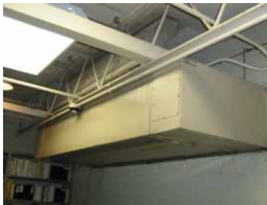
Original Nesbitt ceiling-mounted unit ventilator serving the music storage room
