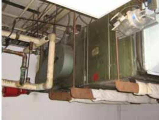
Original AHU located in custodial break room serving B106 and B108 and the ancillary offices
