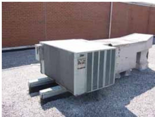
One of (2) Trane RTUs serving the main offices
