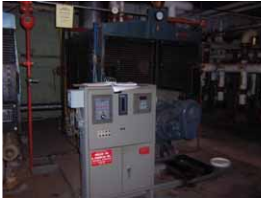
One (of 3) HB Smith Boilers in the original boiler room
