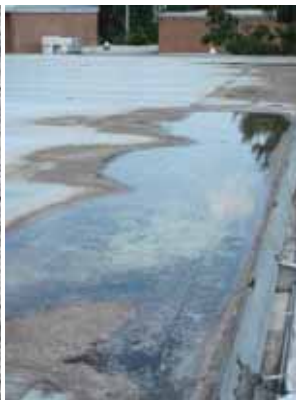
Signs of standing water/pooling
