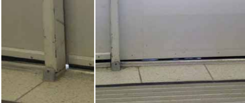
Missing/worn weather-stripping was found throughout the building
