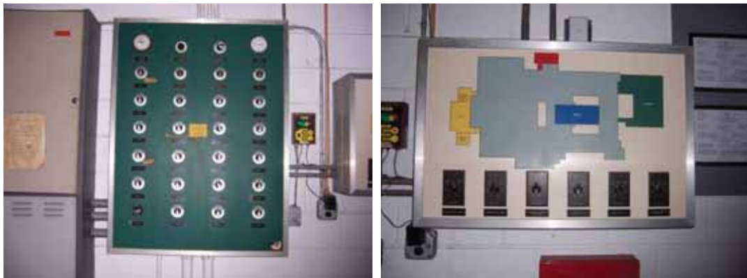
Honeywell Communications Panel (Left) and Johnson Control Panel added during a 1980's addition
