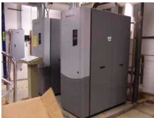
(2) Aerco benchmark boilers in the 2002 D Wing boiler room
