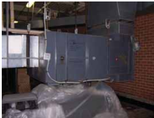
One (of 2) AHUs serving the small gym
