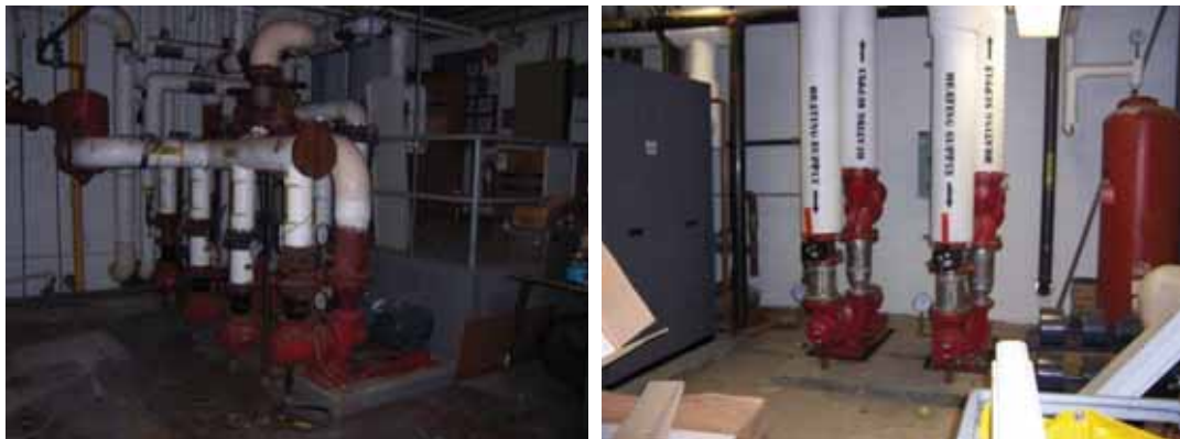
Examples of pumps in the original boiler room (Left) and in the 2002 boiler room
