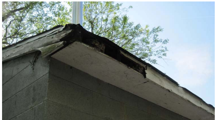
Roof deck deterioration
