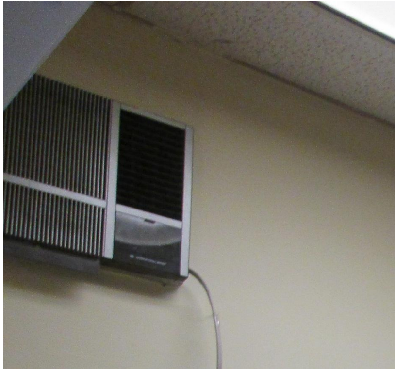
5. Wall Air Conditioning Unit
