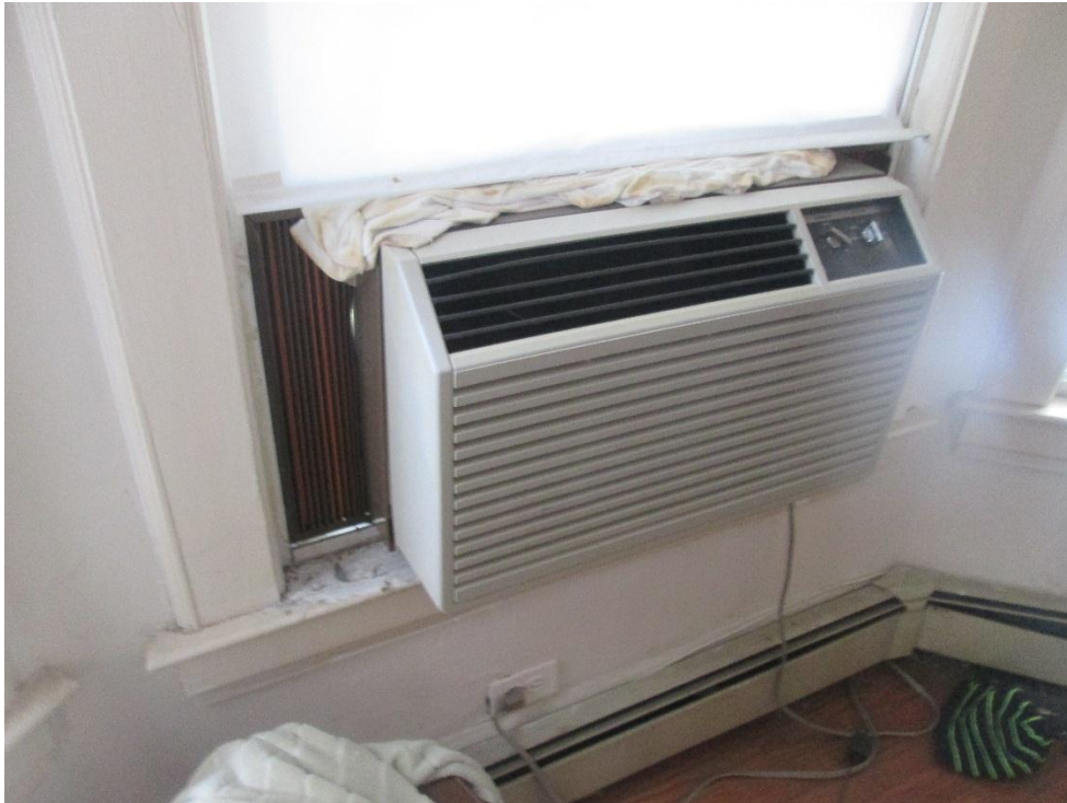
3. Window Air Conditioning Unit
