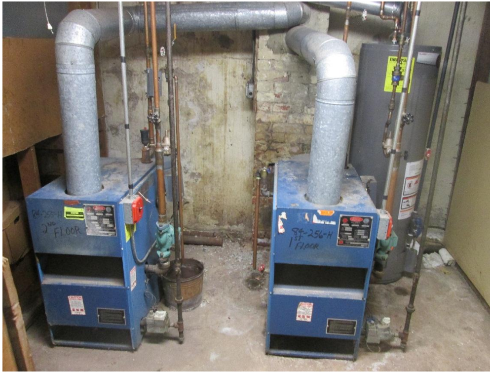
1. Boilers and Hot Water Tank
