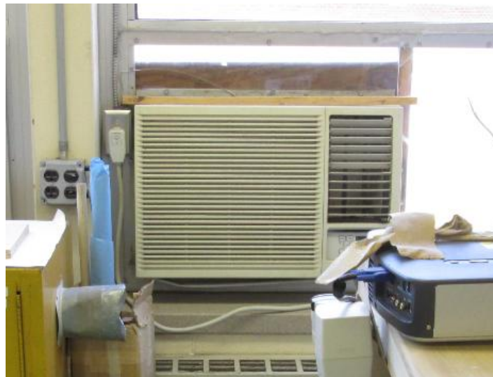
5: Window AC unit Industrial Arts wing
