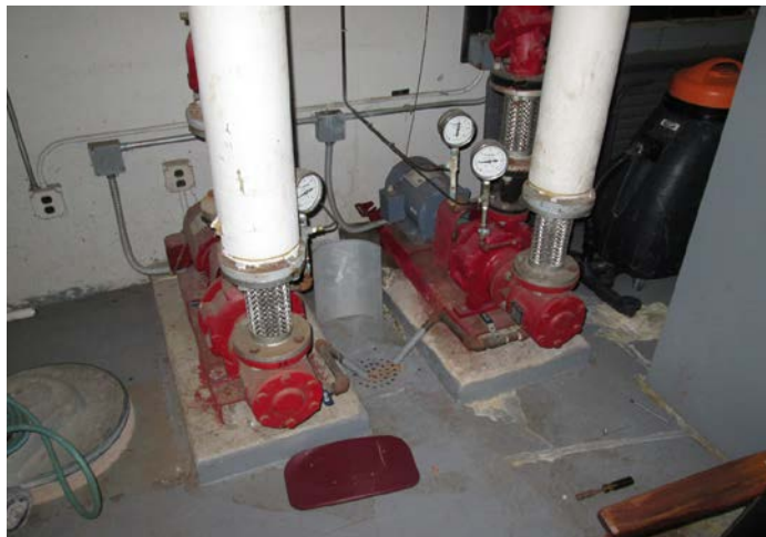
2: Hot water system pumps w/o VFDs
