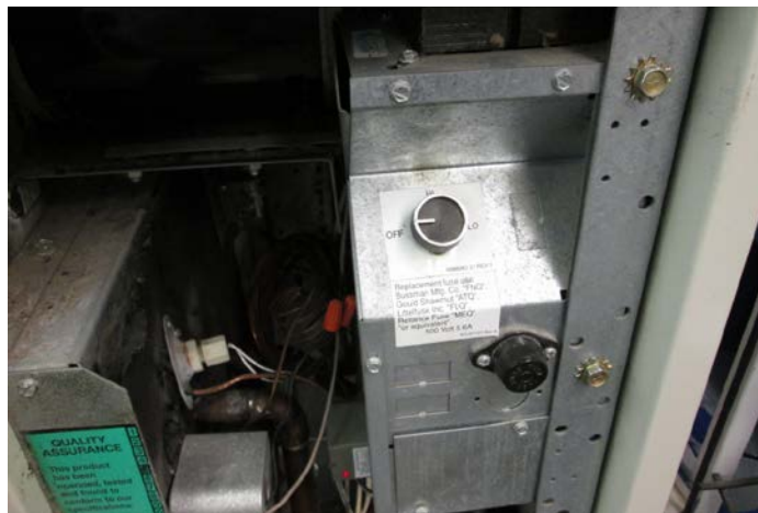
3: Classroom unit ventilator manually turned off
