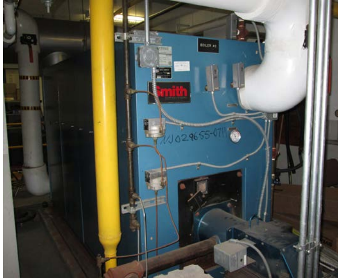
1: Hot water boiler
