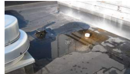
Pooling on Roof
