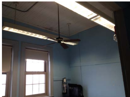
L1: Example of existing lighting in classroom
