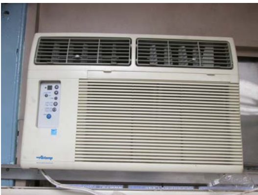
3: Existing window AC unit
