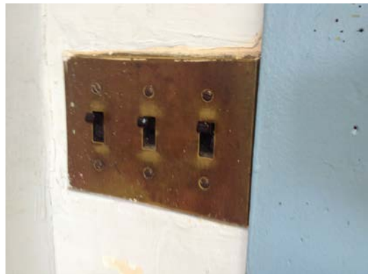
L2: Example of existing lighting controls
