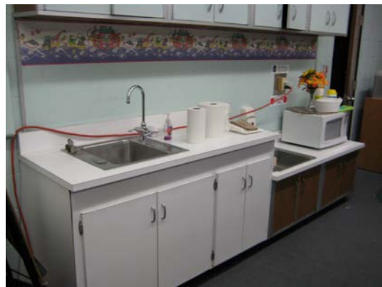
7: High flow faucets
