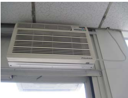
2: Typical window a/c unit
