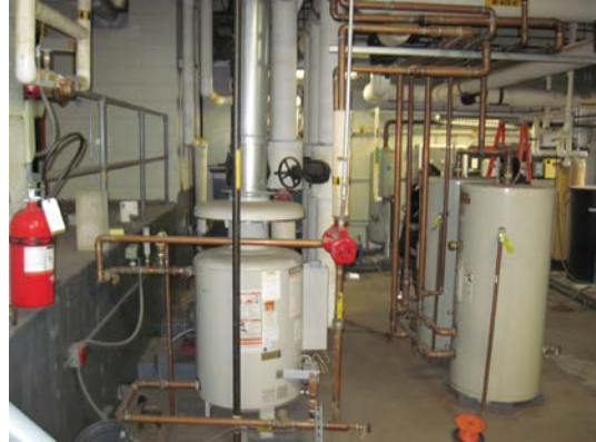
6: Existing DHW Heater
