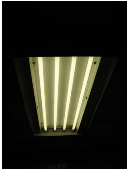
L1: Example of existing lighting in classroom
