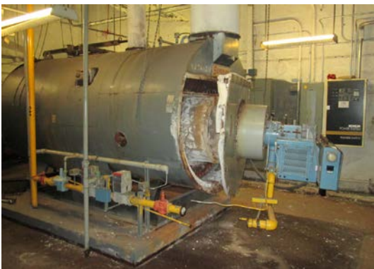
2: Aging steam boiler at Franklin
