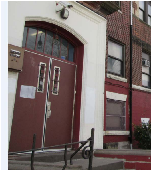
1: Gap in allows for air infiltration
