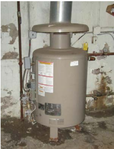
5: Gas-fired DHW boiler
