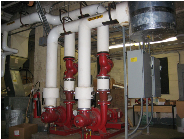
2: Heating hot water pump motors
