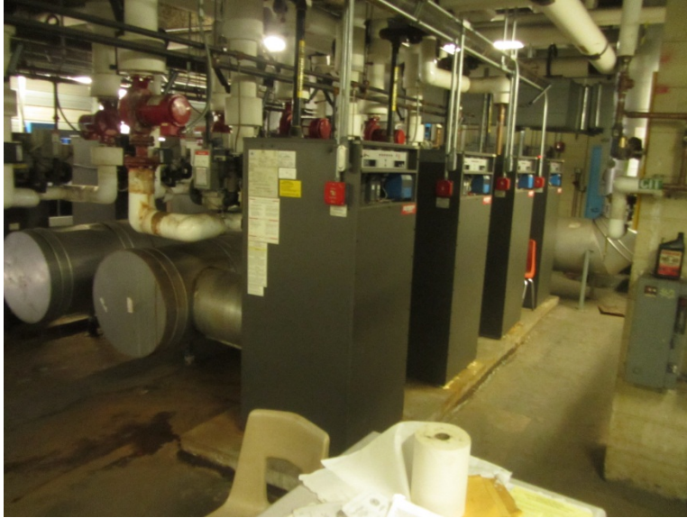
1: Existing hot water boilers (7 total)
