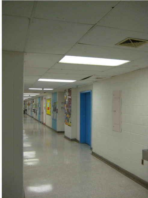
7: Sample corridor lighting fixtures
