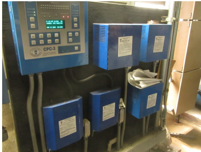
4: Boiler controller system
