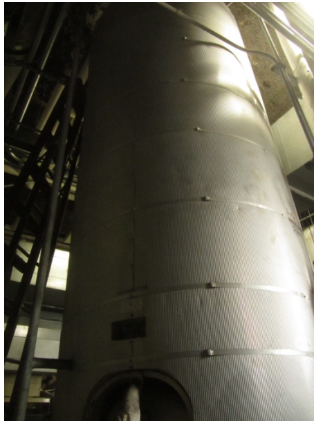
6: DHW storage tank
