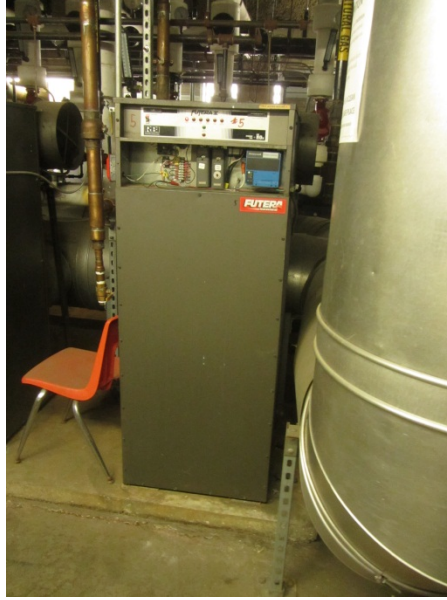
5: Domestic hot water (DHW) boiler
