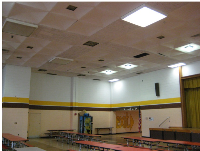
8: Sample multi-purpose room lighting fixtures
