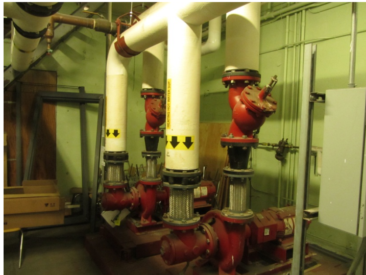
2: 20 HP Hot water pump motors
