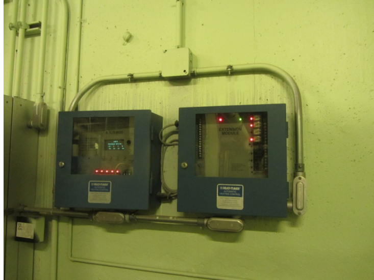
3: Existing boiler controls
