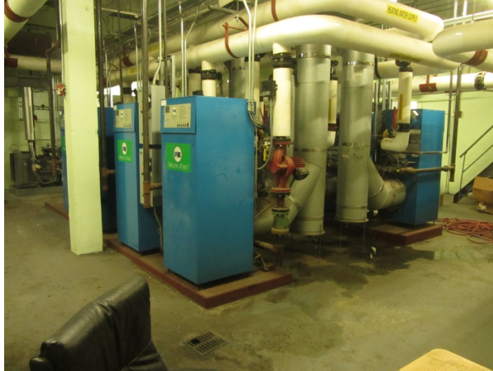
1: Existing heating hot water boilers
