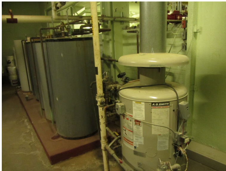
4: DHW boiler with storage tank bank
