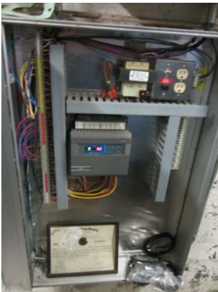
3: Existing boiler control system
