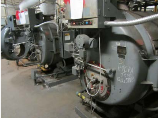
1: Existing steam boilers in building
