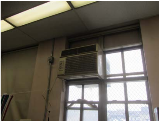
2: Typical window a/c unit
