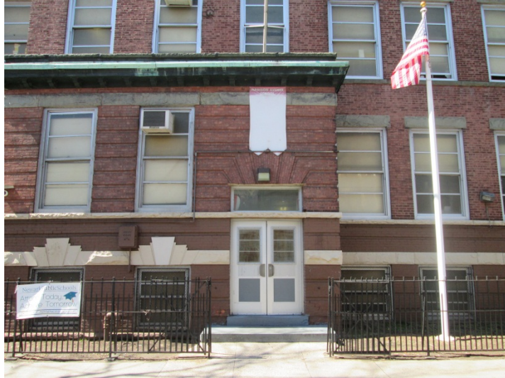
1: Gap present between doors
