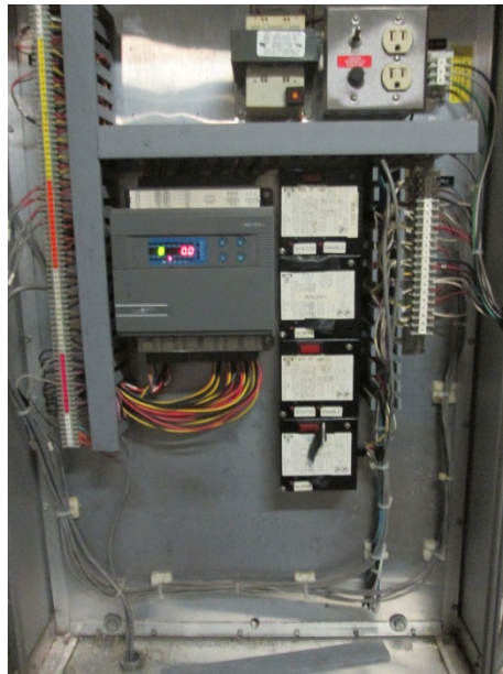
4: Johnson Metasys controls system
