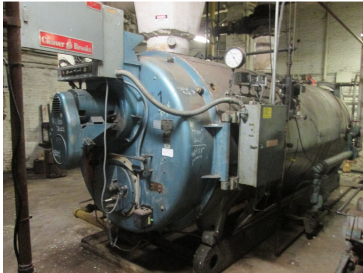
2: Existing steam boiler
