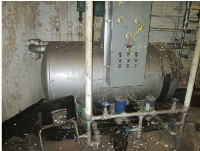
3: Steam boiler condensate return tank
