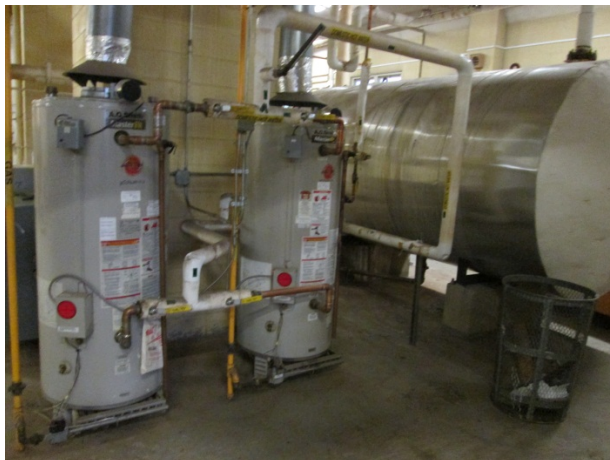
5: Existing DHW generation equipment
