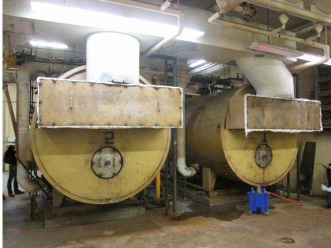
1: Existing steam boilers
