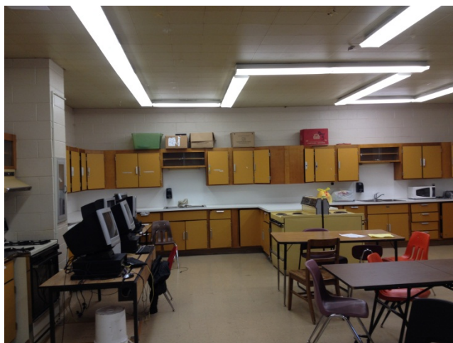
6: Typical classroom lighting fixtures
