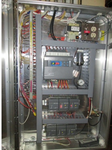
4: Johnson Metasys controls system
