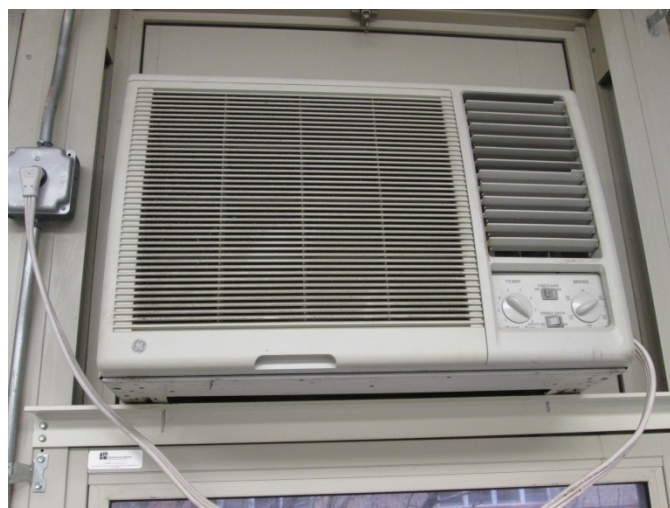
3: Typical window AC in building
