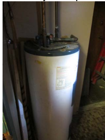
4: One of two electric DHW heaters in building
