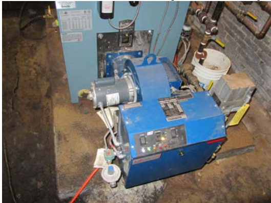
1: Existing oil burner
