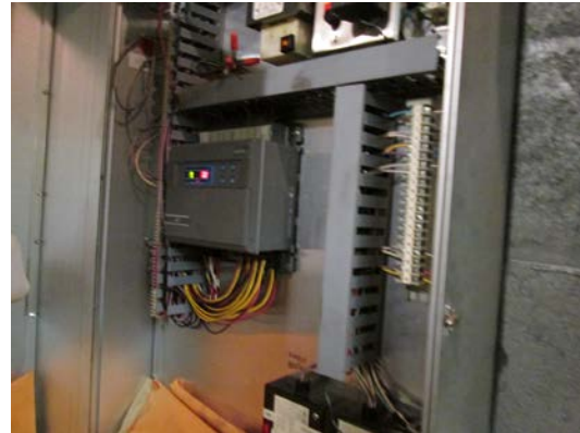
3: Existing boiler controls
