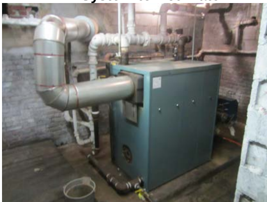
2: Steam boiler located in basement
