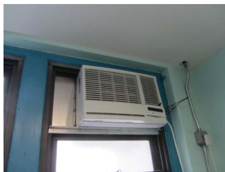
3: Typical window a/c unit
