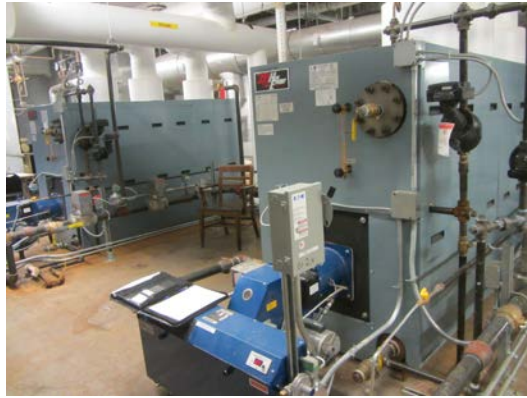
1: Existing steam boilers located in boiler room
