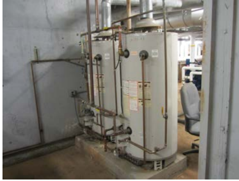
4: Existing DHW system
