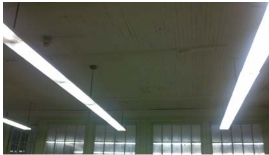
6: Example of existing lighting in classroom
