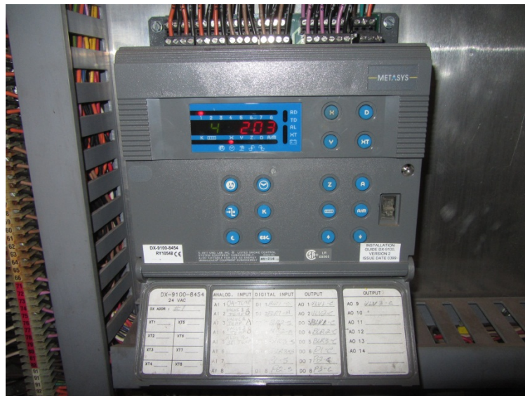
4: Johnson Metasys controls system
