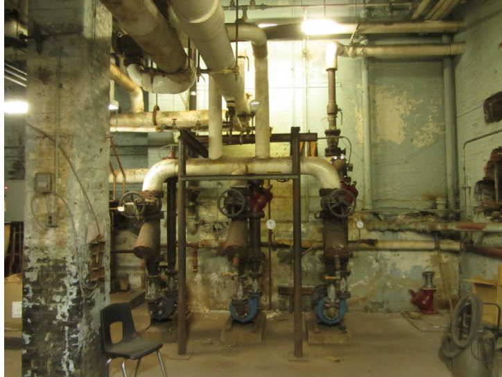
3: Example of pumps in boiler room
