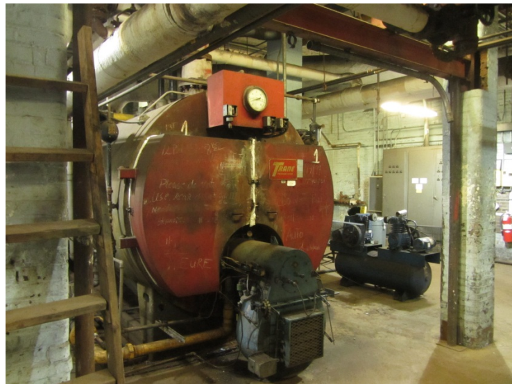
2: Example of steam boiler (one of three)
