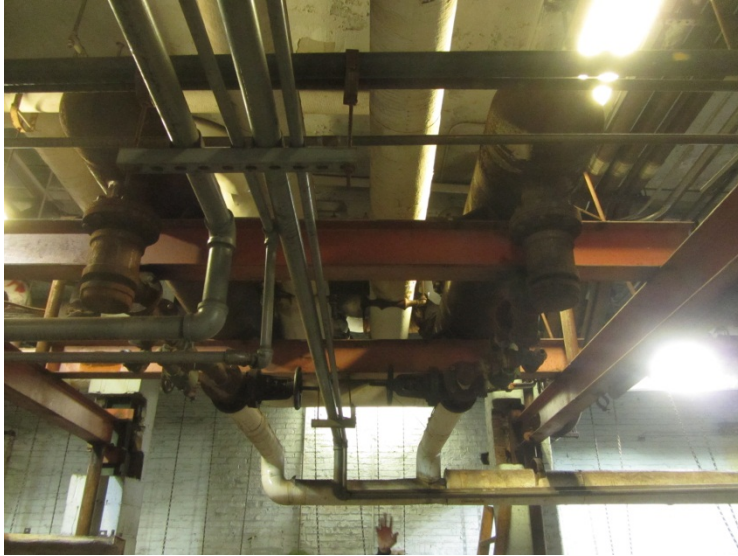
1: Existing steam to hot water heat exchangers
