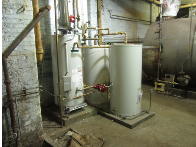
5: DHW heater and storage tanks
