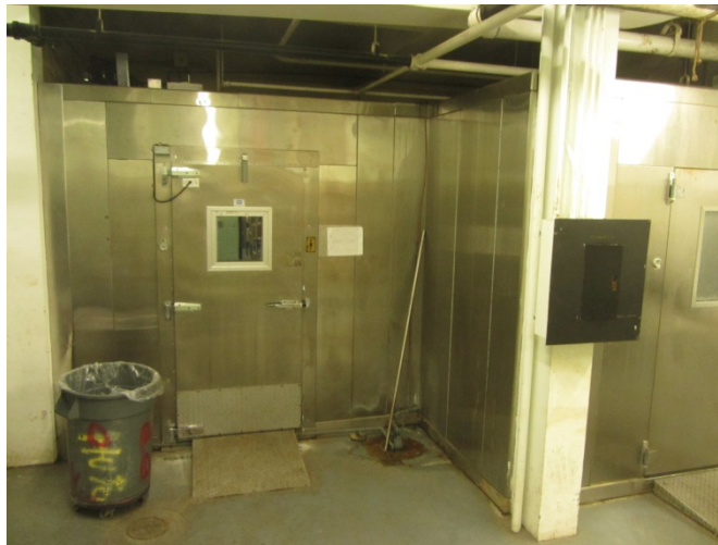
6: Walk-In cooler unit in basement under kitchen
