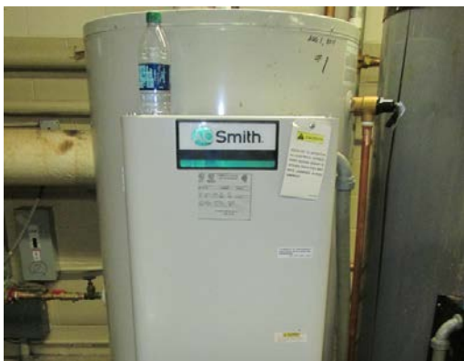
3: A.O. Smith 45000 watt electric DHW heater
