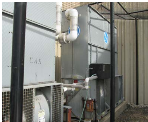
6: Two BAC cooling towers
