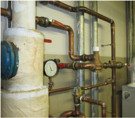
2: Un-insulated DHW piping
