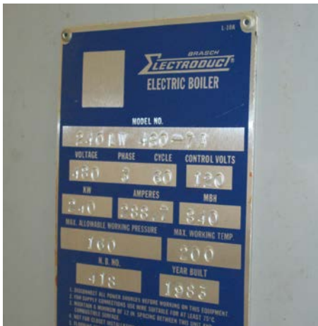
1: Electroduct electric boiler should be replaced
