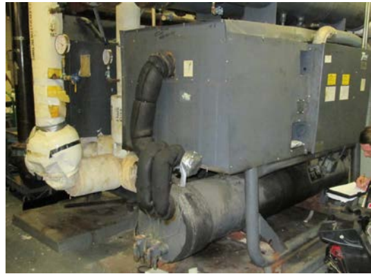
4: Existing chiller in mechanical room
