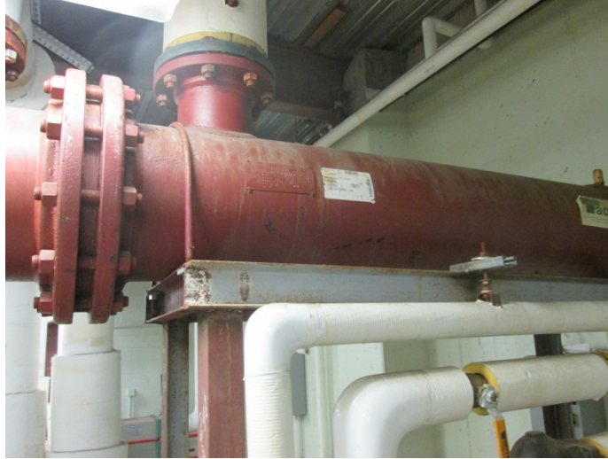
1: Existing Heat Exchanger
