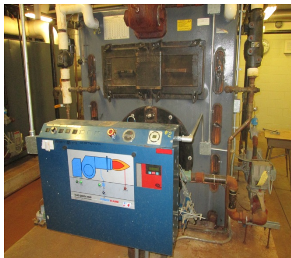
3: Existing Steam Boiler
