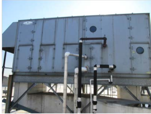
4: Existing Energy Recovery Unit
