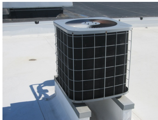
5: Existing Condensing Unit
