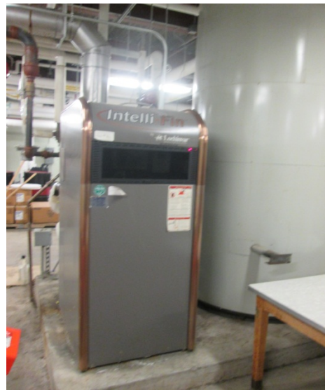
2: Existing Domestic Hot Water
