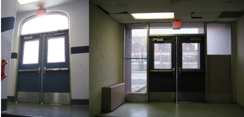
1: Visible gap around door edges
