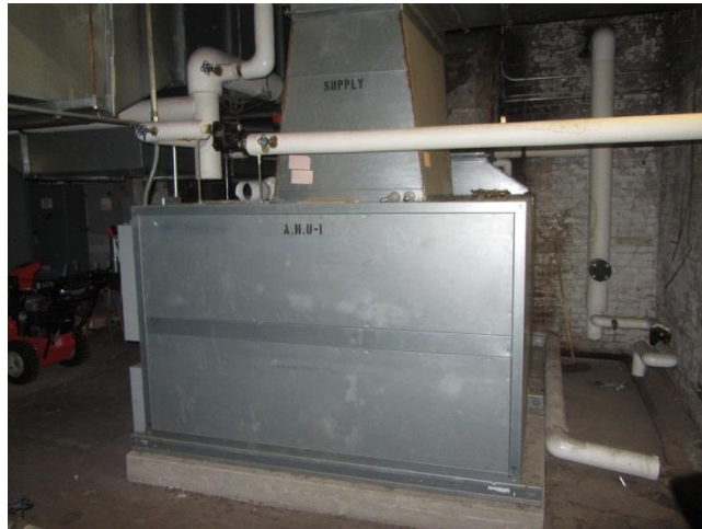
5: Heating and Ventilation (HV) unit in fan room
