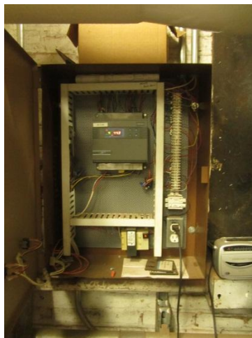
6: Johnson Metasys controls system
