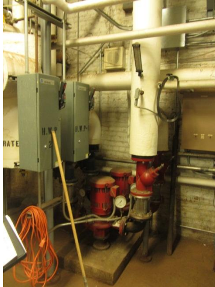
4: Hot water pump motors
