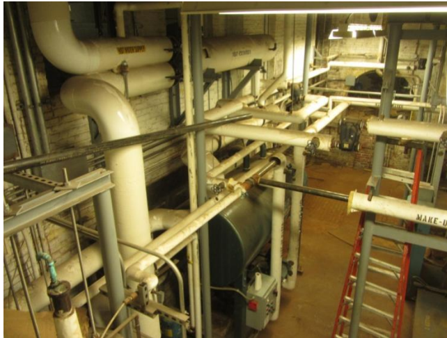
2: Existing hot water heat exchanger
