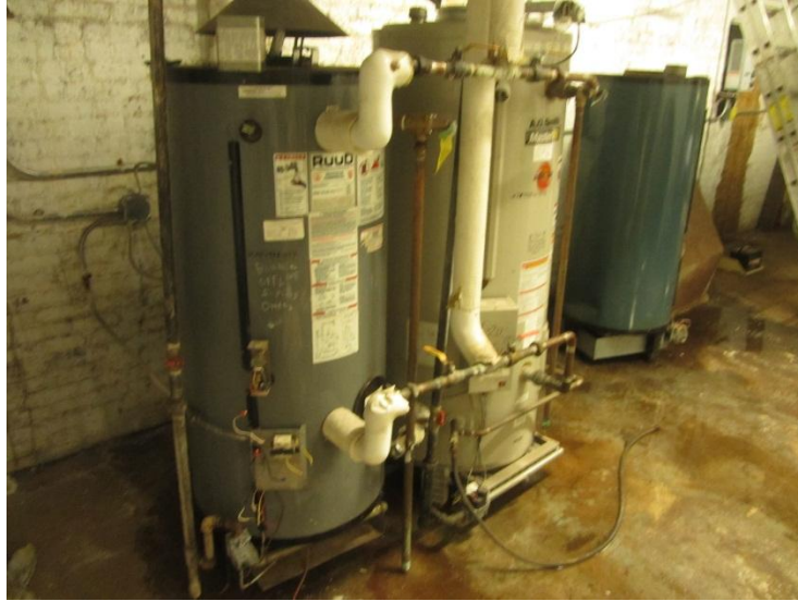
7: Domestic hot water (DHW) heaters
