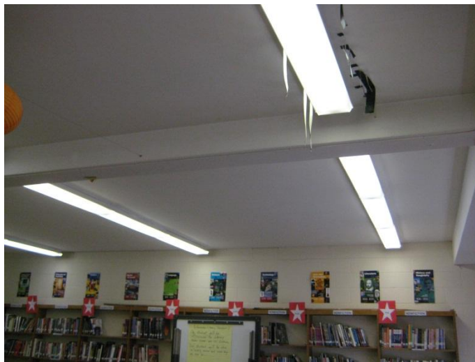
8: Example lighting fixtures in media center
