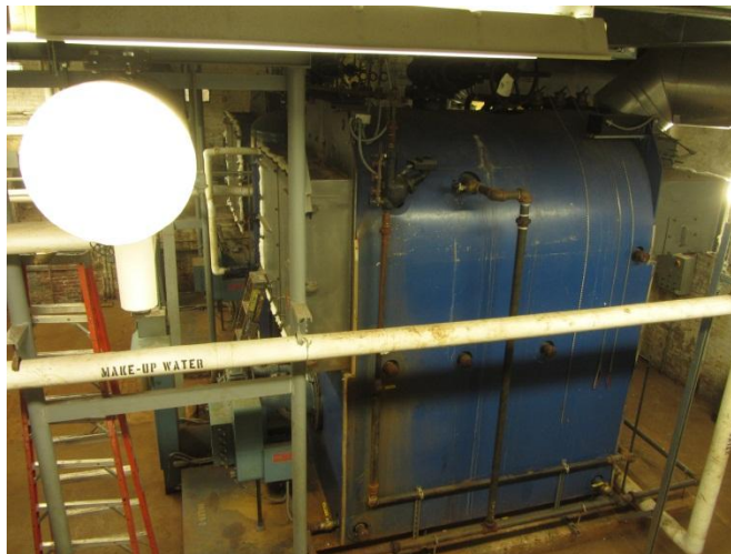
3: Existing steam boilers
