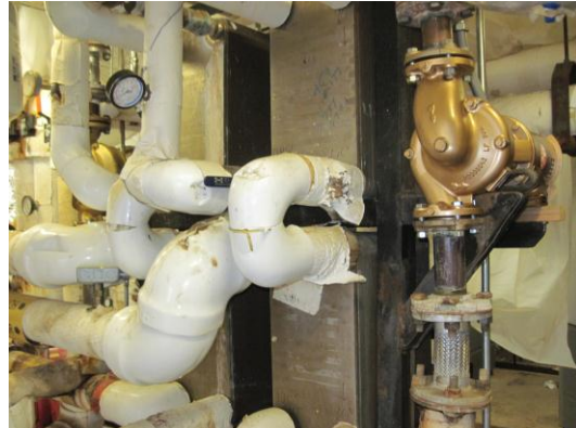
Existing Heat Exchangers
