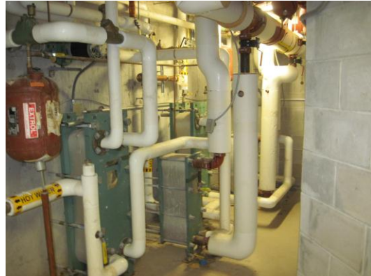
Existing Heat Exchangers
