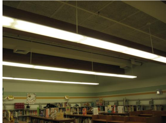
Existing T8 Lamps
