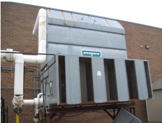
Existing Cooling Tower
