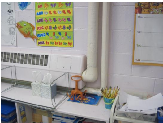
Existing Steam Radiator
