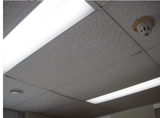
Existing T8 Lamps
