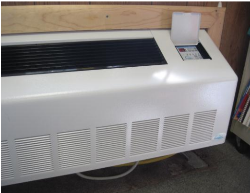
Existing PTHP Unit
