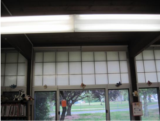
Existing T12 Lamps
