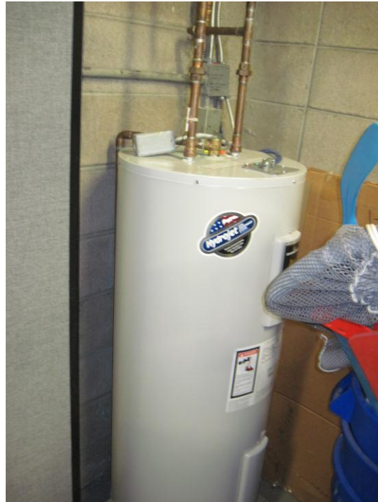
Existing DHW Heater
