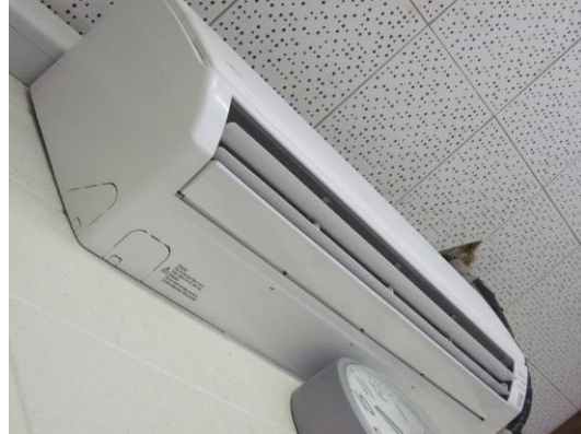
Existing Split Units
