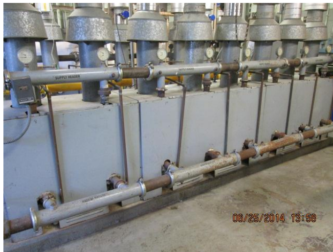
2: Hydrotherm modular hot water boilers
