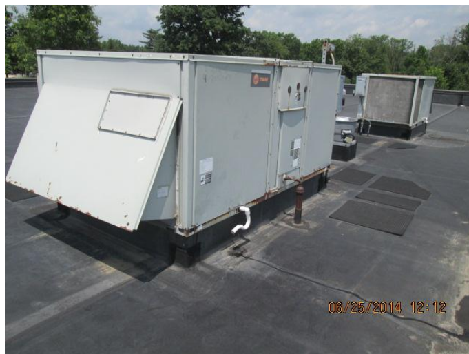
3: Trane rooftop units
