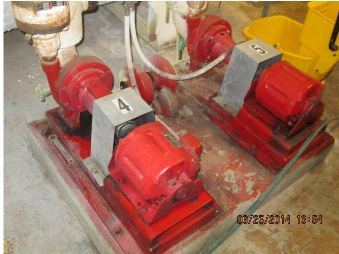
4: Base mounted hot water pumps
