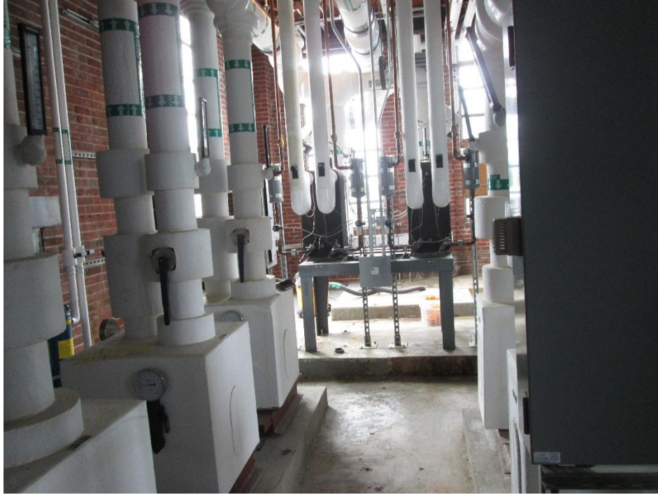
5. Chilled water pumps and heat exchangers in 1958 tower
