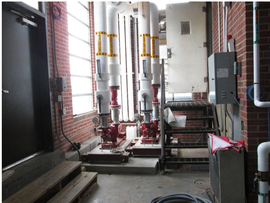
4. Hot water pumps in 1958 tower
