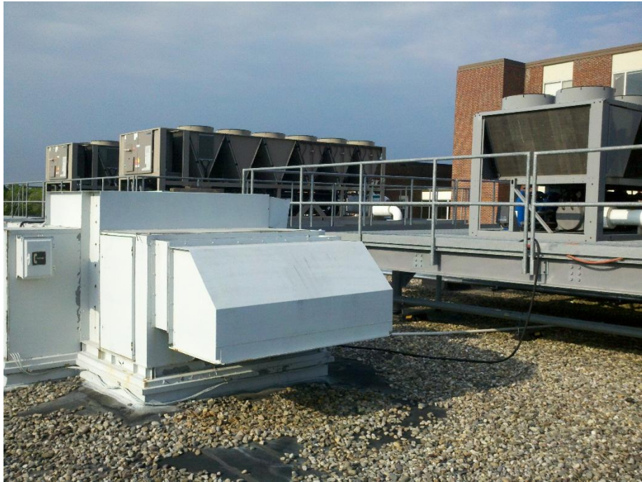
1. Existing Air Cooled Chillers and Air Handler on 1978 Roof
