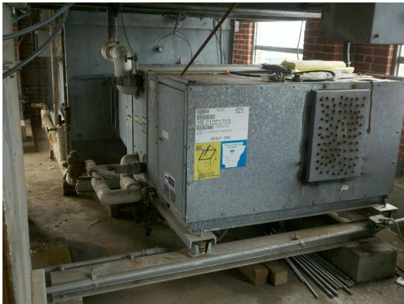
2. Air Handler in 1958 Tower
