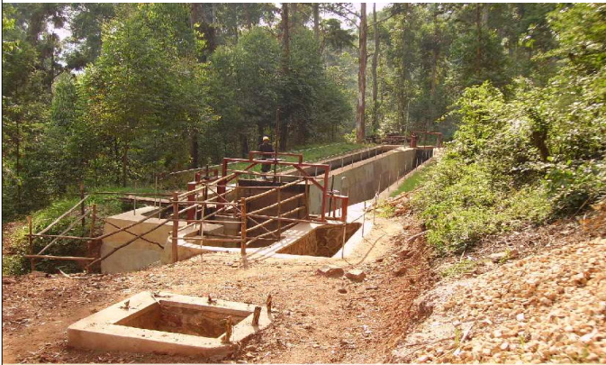
60 kW and 300 kW supply channels and de-silting tank and gates
