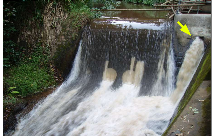
The reserve flow - arrowed - is now ensured.
