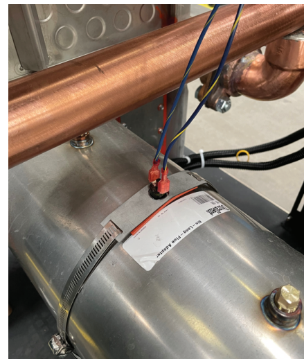
Figure 4. Installed Vent Limit Switch
