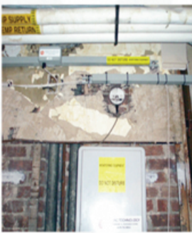
One of the sensors used to monitor building movement during demolition and pile driving.
