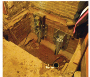
Hydraulic ram pressure testing pile (left), and a pile driven and secured in place.
