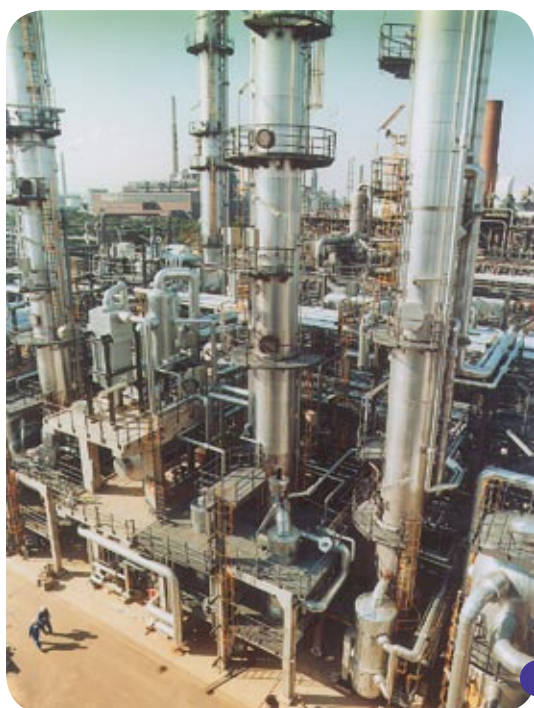
FIGURE 189: Plant for obtaining ethylene, the raw material used in the production of polyethylene (BASF factory photo, Ludwigshafen, Germany).
