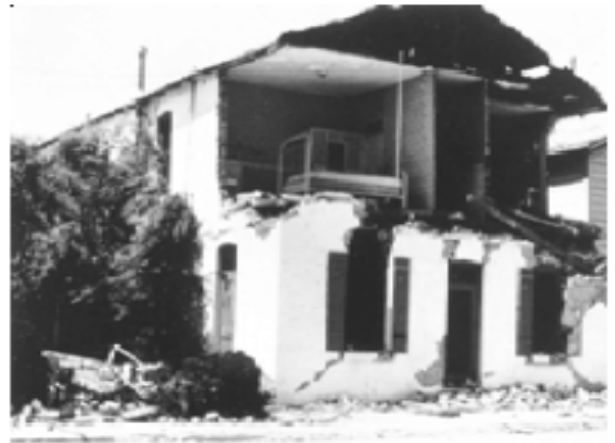
Figure 25 - The plaster-covered brick walls of this building collapsed during a recent earthquake.
