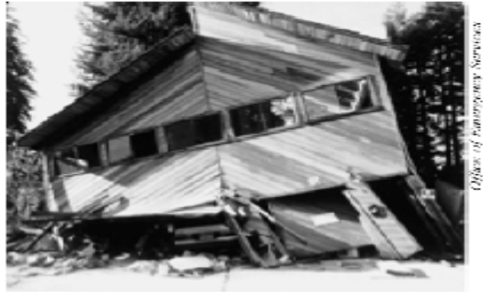
Figure 29 - This mountain home was built over a garage, and its walls were not strong enough to withstand an earthquake.
