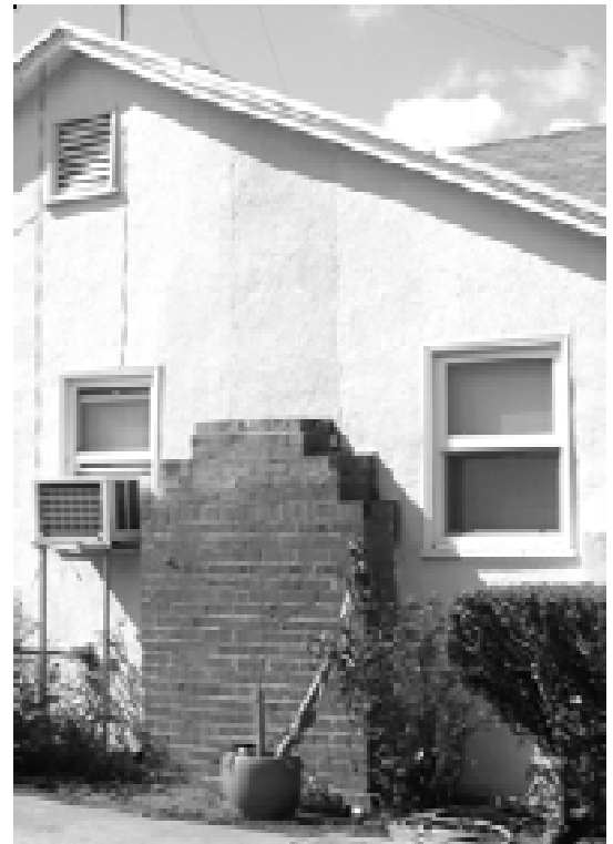
Figure 35 - Photo showing damaged chimney removed. Note that the fireplace is now not functional.
