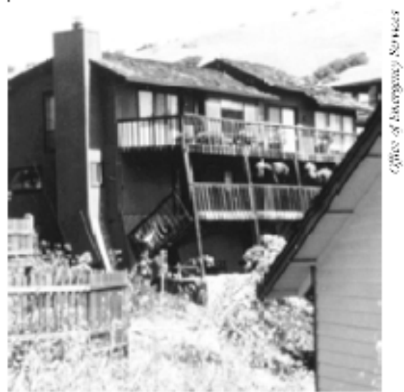
Figure 22 - This hillside home was built on an unbraced tall wall that failed.
