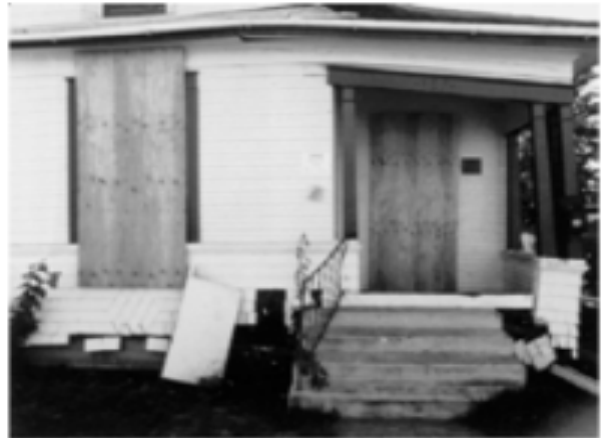
Figure 13 - This home wasn't bolted and slid off its foundation. Sometimes the damage can be so bad that houses have to be demolished.
