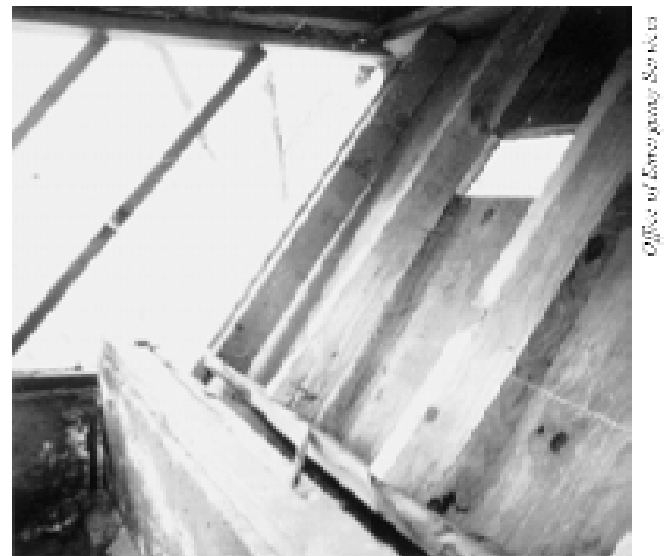
Figure 23 - This photograph shows an interior detail of a home similar to the one above, showing substantial damage to a building with an unbraced tall wall.
