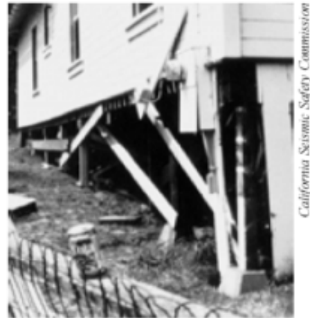
Figure 18 - The pier-and-post foundation under this home shifted during a recent earthquake.
