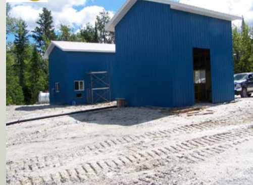
Foley Mine - New construction on collar of North Shaft to permit underground exploration.
