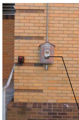
ELIMINATE FIRE ALARM PULL BOX (PENDING)
