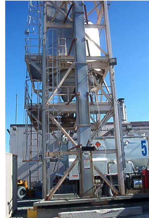
Ammonium Nitrate (AN) Silo
