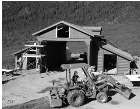
Midcamp looks a bit different with the raising of a timberframe barn!
