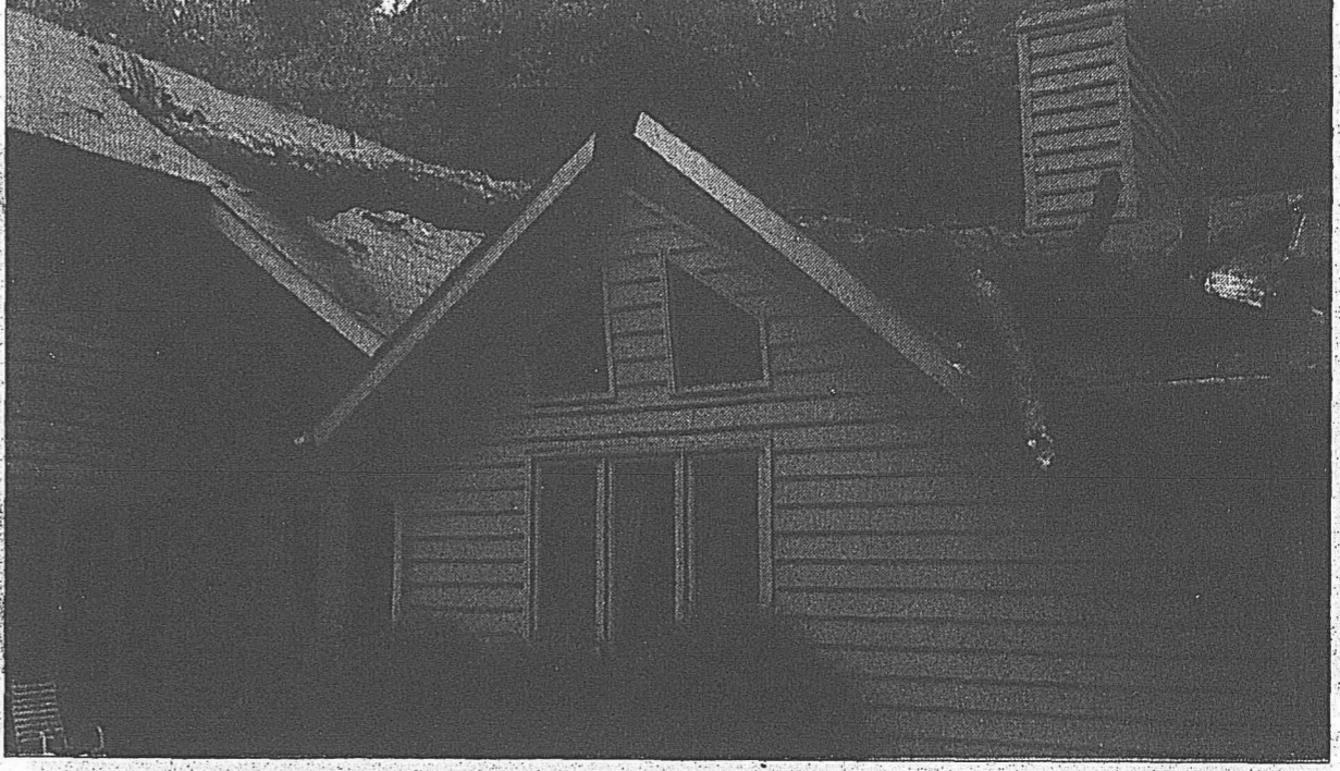
Awakened in the early morning hours by a severe thunderstorm, the Brandermill residents moved from their upstairs bedroom moments before a tree crashed through their roof. The August 5 storm caused damage from fallen trees in at least five Brandermill neighborhoods.
