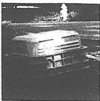
Photo by Janet Joyce Comcast Cablevision is installing numerous "cat houses" throughout the community. They house fiber optic equipment. Some highly visible cat houses may be screened.
