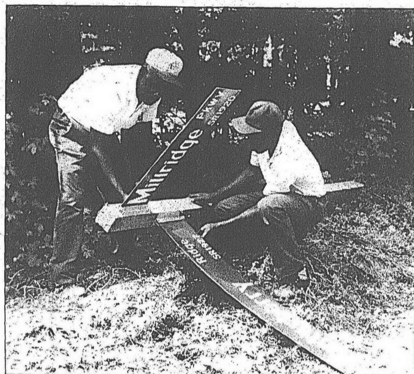
Photo by Wendy Parker BCA employees Garland Bannister and Brad Mitchell repair three street signs which had been vandalized in Winterberry Ridge. Cost of materials and labor in replacing each post is about $75. (See Reward Box.)
