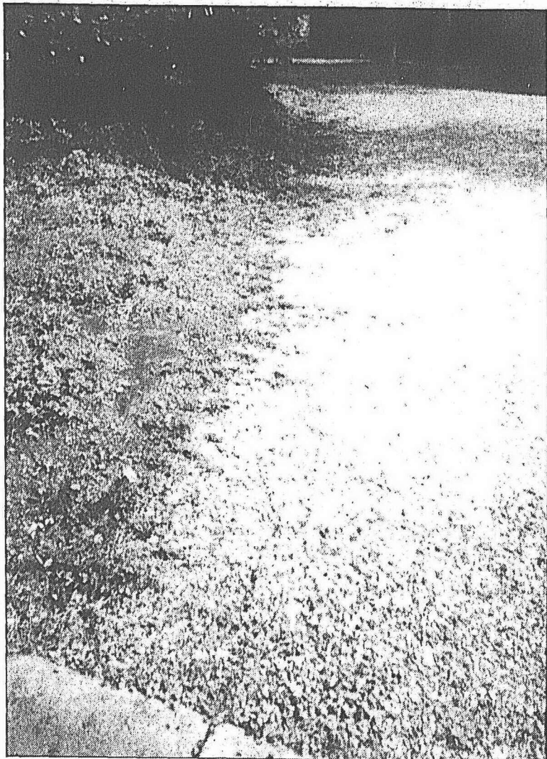
An undefined driveway looks unkempt.
