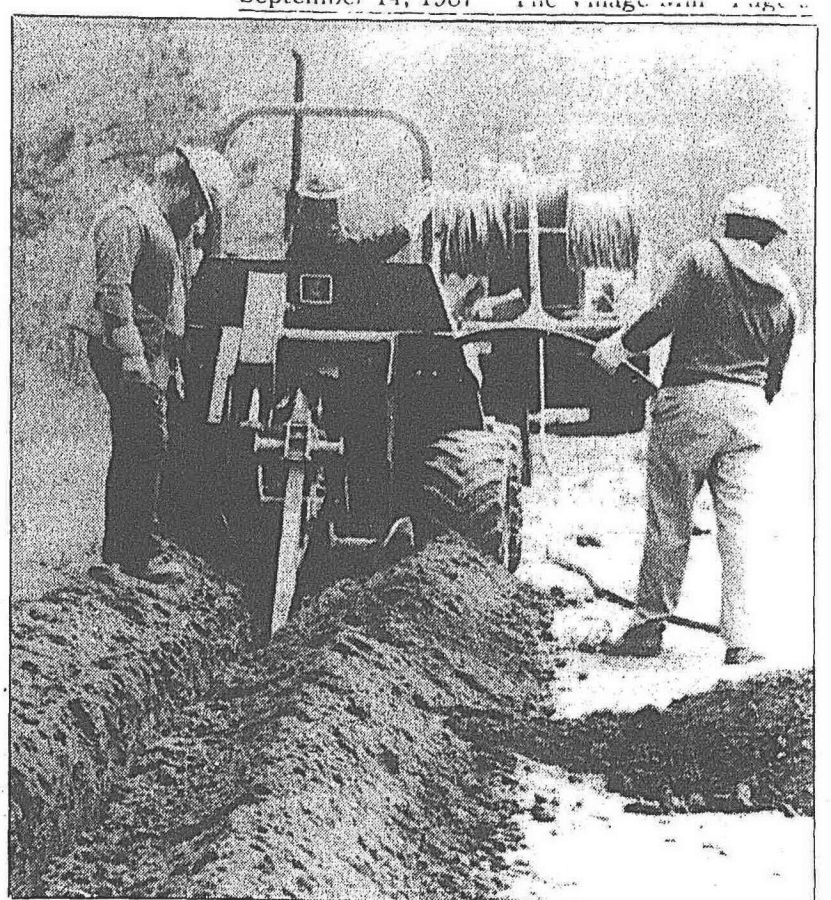
Virginia Power workers have been busy replacing underground cable in Brandermill. In 1987 13,600 feet of cable will have been replaced.
