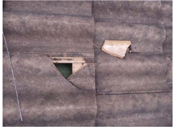
Damaged roof tiles
