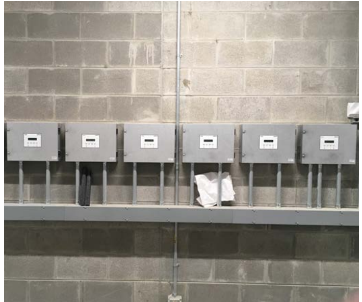
EBC30 Controllers are used for the Modulating Overdraft Dampers
