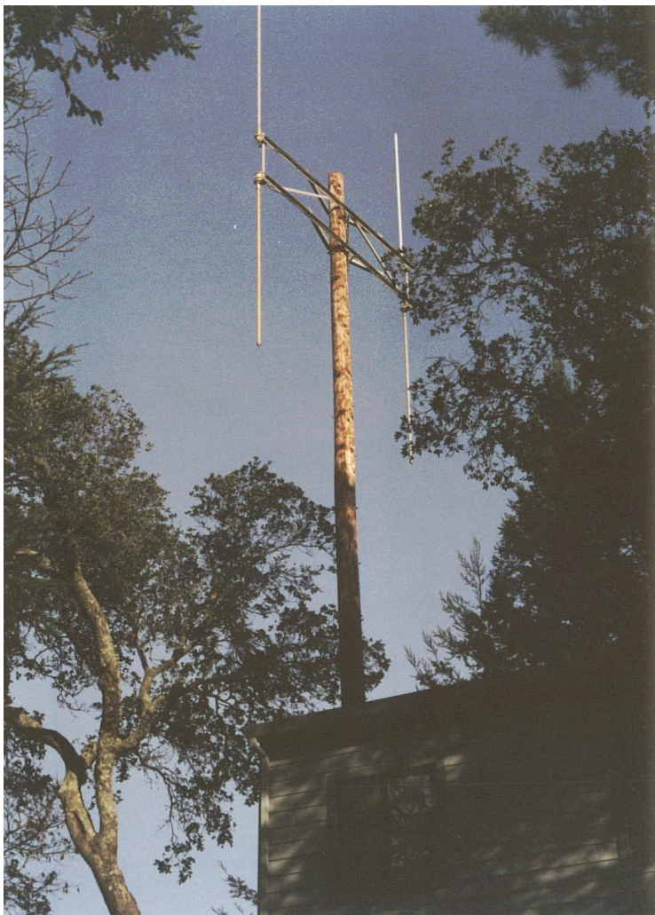
Two whip antennas at a Cellular site in California.
