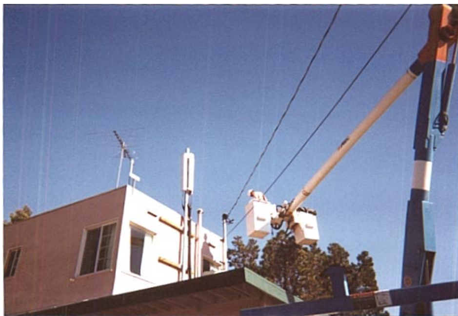
Dual-polarized personal wireless service facility being installed on the second floor of a motel in Marin County, California
