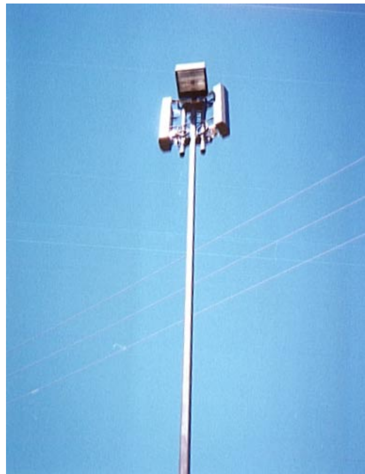
This personal wireless service facility has two dual-polarized antennas with a single floodlight.
