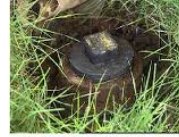
Typical sewer cleanout with properly installed plug.
