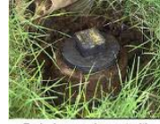
Typical sewer cleanout with properly installed plug.
