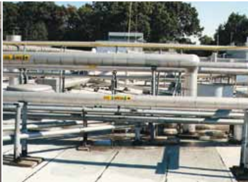
Excessive Roof Loading
