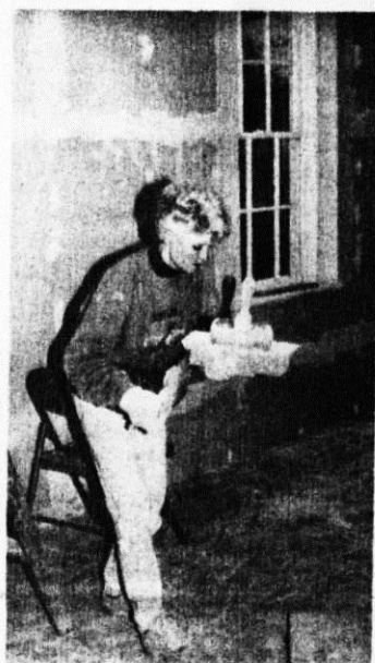
Paula Garber prepares dry-wall mud while working on the Robert E. Jones Hall as part of a work team from Lake Junaluska.
